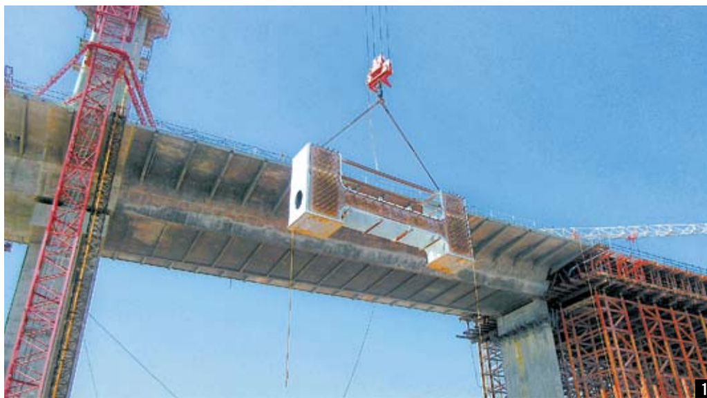
1 Lifting a cable anchor box, 2 A worker working on cable installation, 3 Installation of key segments from January 25 to 26.
